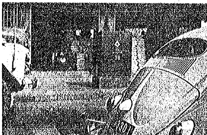
Installation position of cross-connecting cabinet (type 600).
