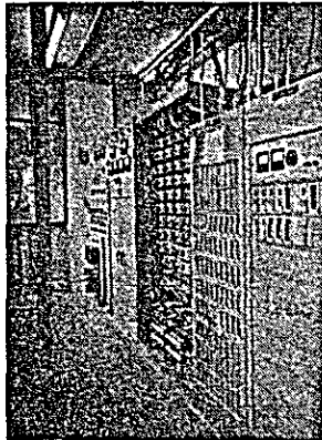
Fig. 4-7-53 Signal apparatus room
