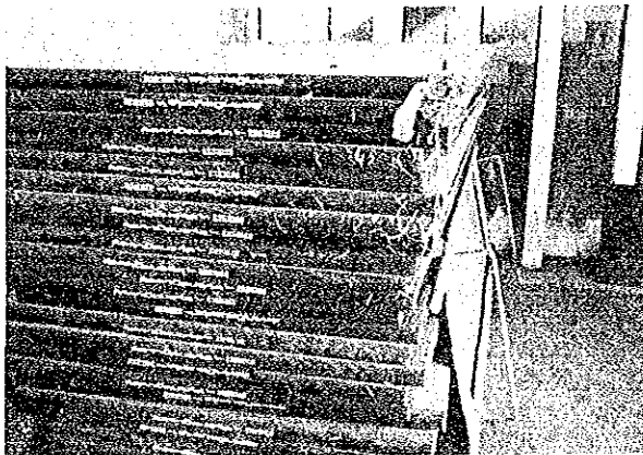
Asbesto-ceiling with insulation board
