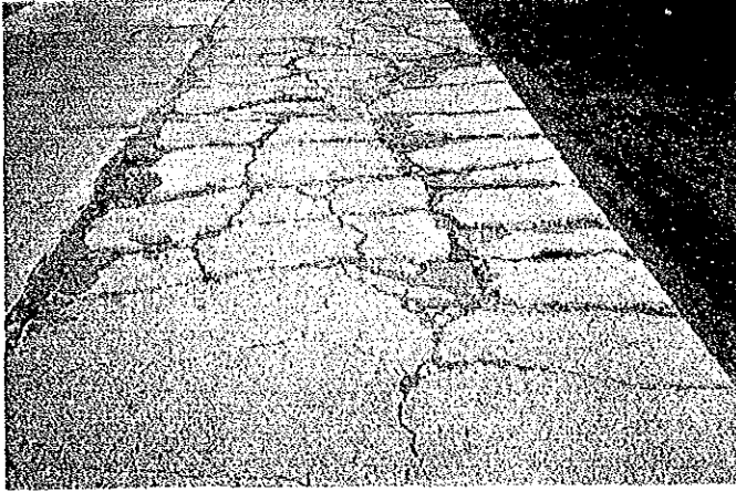
BLOCK CRACKING (Separation of Slab)
