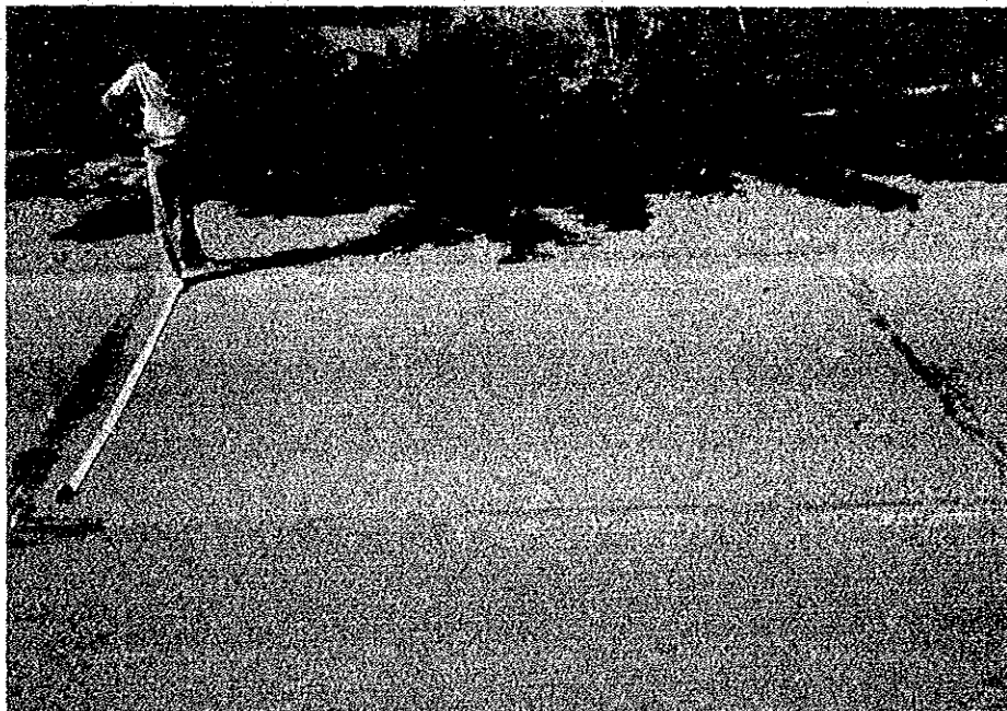
FIGURE 8.2-2 (1) DETERIORATION CONDITION OF N 2 -G SLAB
