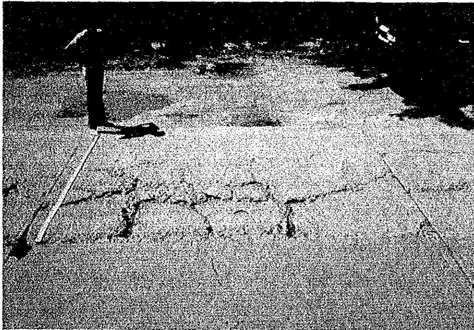
FIGURE 8.2-3 (3) DETERIORATION CONDITION OF N 3 -B SLAB
