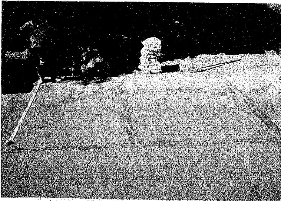
FIGURE 8.2-2 (3) DETERIORATION CONDITION OF N 2 -B SLAB
