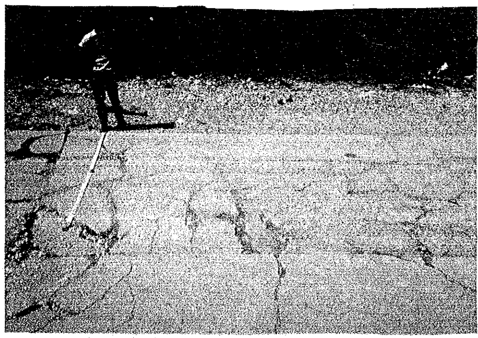
FIGURE 8.2-5 (3) DETERIORATION CONDITION OF S 2 -B SLAB
