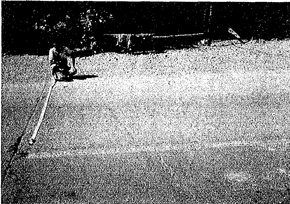
FIGURE 8.2-2 (2) DETERIORATION CONDITION OF N 2 -F SLAB
