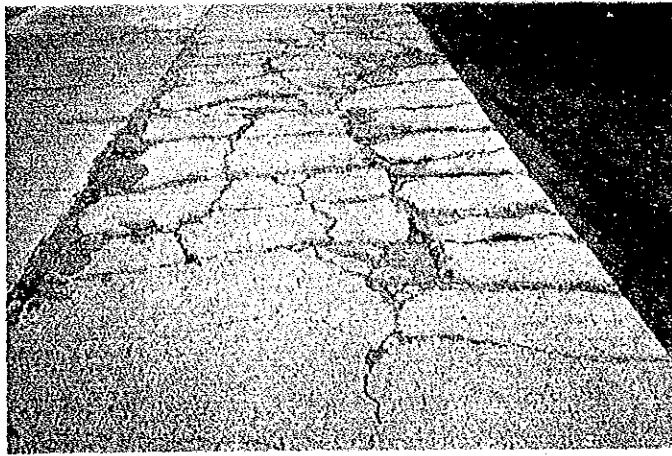
BLOCK CRACKING (Separation of Slab)
