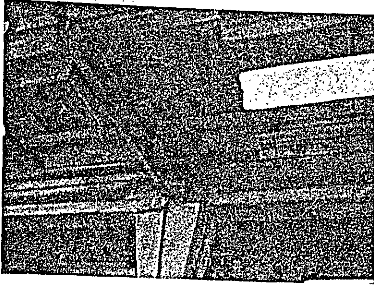
Photo 5.80 A one-story plant of precast, prestressed construction, Bucharest. (Cast-in-place columns; 6 m in story height; the natural period, about 1.5 seconds; slightly damaged)
