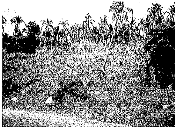
LANDSLIDE SOIL LANDSLIDE L.S (S)
