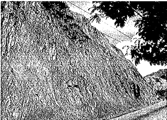
CUT SLOPE SURFACE FAILURE (WEATHERING) C-S.F (W)
