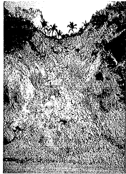
CUT SLOPE DEEP FAILURE (SCOURING) S-D.F (S)
