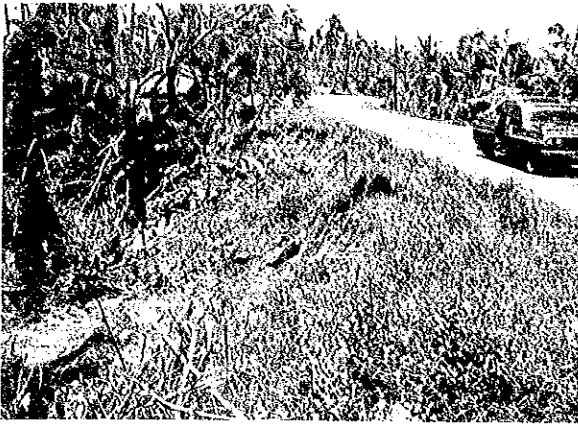
EMBANKMENT SLOPE MAHARLIKA HIGHWAY, SURFACE FAILURE SOUTH LUZON (EROSION) km 406 + 490 E-S.F (E)
