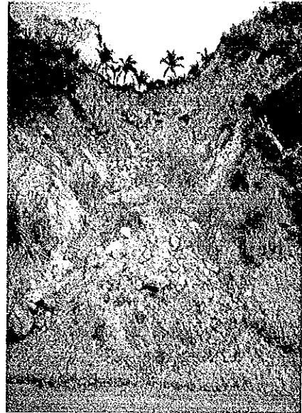
CUT SLOPE DEEP FAILURE (SCOURING) S-D.F (S) MAHARLIKA HIGHWAY, LEYTE km 1019 + 690
