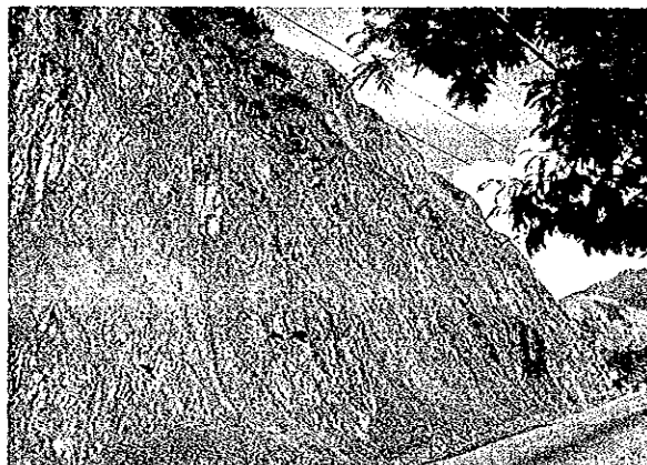
CUT SLOPE SURFACE FAILURE (WEATHERING) C-S.F (W) KENNON ROAD km 237 + 800
