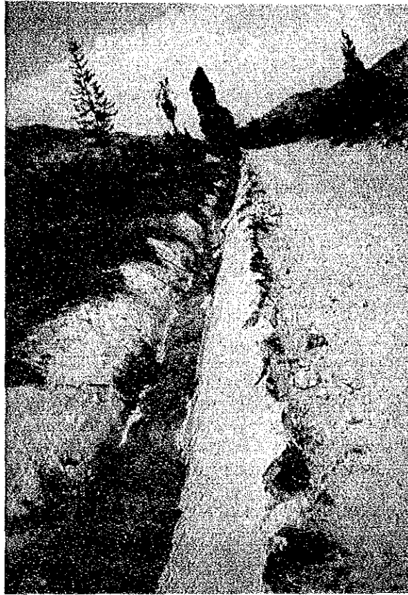
Deteriorated Lining of Irrigation Canal
