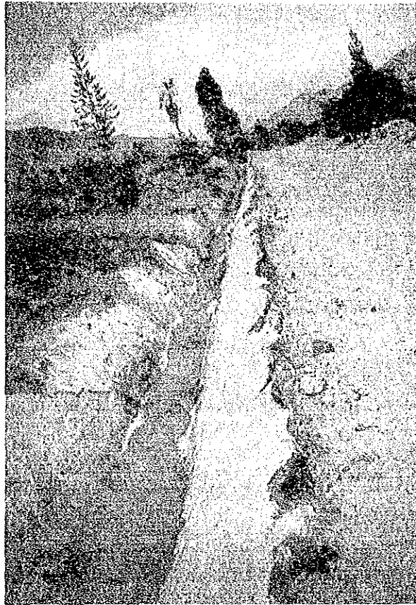
Deteriorated Lining of Irrigation Canal
