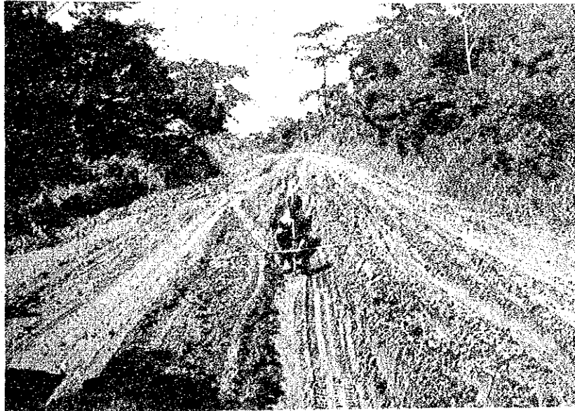
Rutty Road Surface
