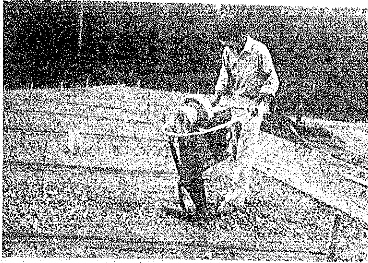
Photo 7: Gravel is spread in its average thickness 5m between cross-boards, then, it is pressed by a roller.
