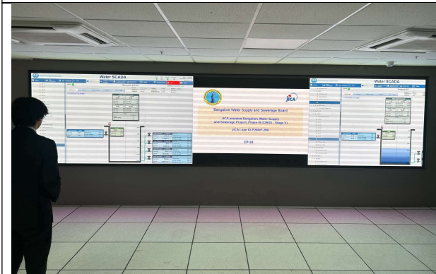
Central SCADA Centre (Bengaluru City)
