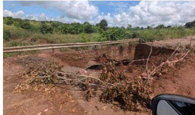
Source: JST Malawi: Road washout on T388 caused by heavy rain (March 2025)
