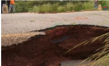
Source: ZNBC Zambia: Road washout on the Great East Road due to heavy rain (January 2025)
