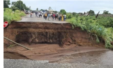
Source: JST Mozambique: Road washout on N12 caused by Cyclone "JUDE" (March 2025)
