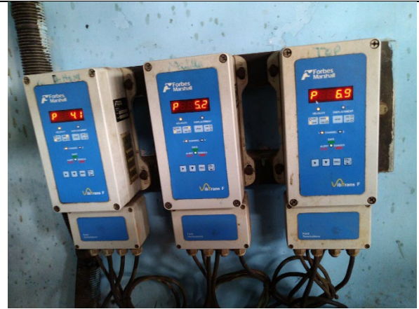
Vibration gauge display (three locations per unit).
