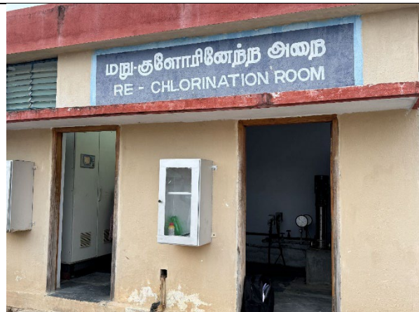
Chlorine Injection Chamber
