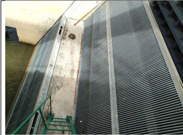
The bar screen has 20 mm spacing, designed to remove debris and protect the pumps.
