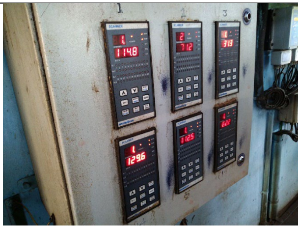
Thermometer indicators for each pump motor, etc. (six stations per unit).
