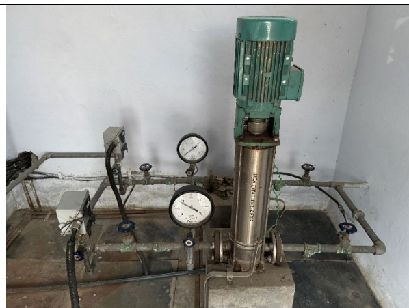
Chlorine Injection Facility and Pumps for Chlorine.
