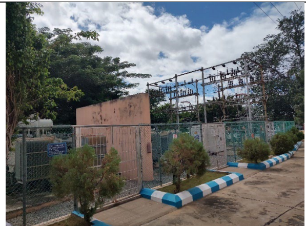
The power receiving equipment consists of two incoming lines operating at 33 kV.
