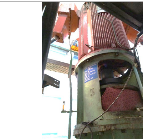
Vibration sensor (three locations per unit).
