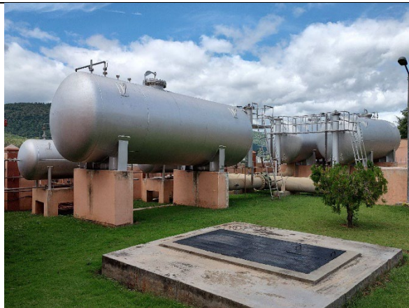
A surge tank is installed to prevent water hammer effects during power failures.
