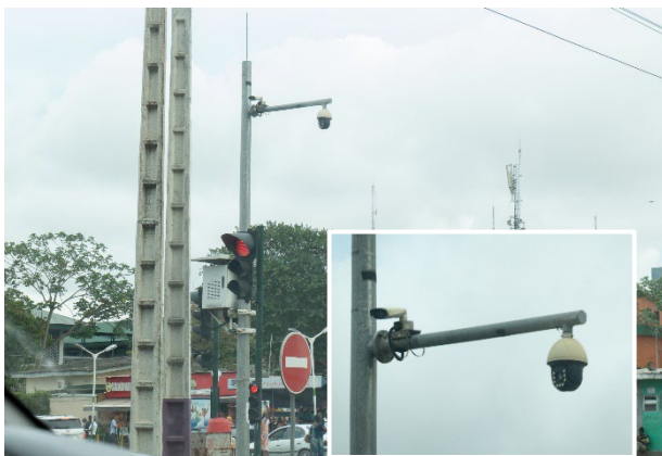
Omnidirectional surveillance camera installed on a general road
