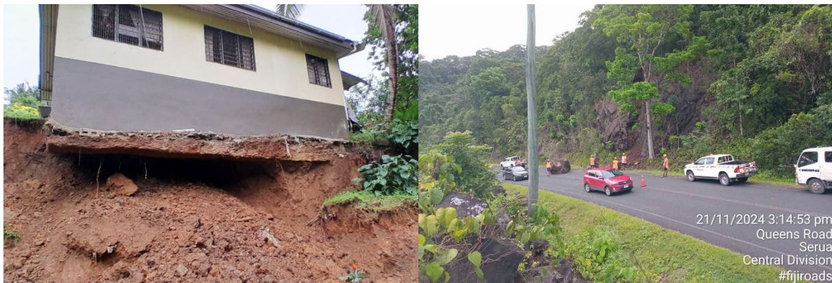
Houses damaged by collapse of steep slope (in Suva City)
