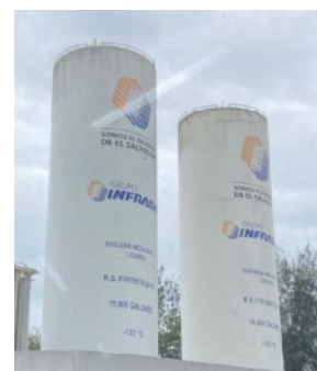
Oxygen tanks (photo by the evaluator)
