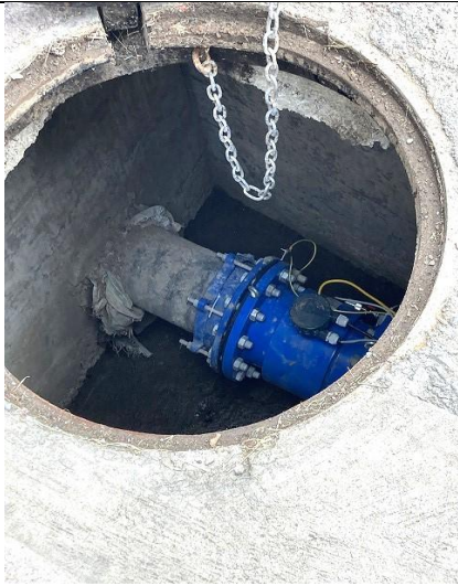
Installed Electromagnetic Flow Meter
