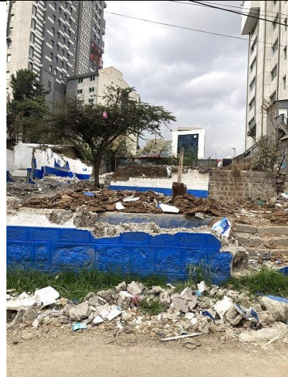
House Damaged by the Corridor Project
