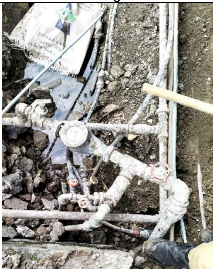
Customer Meter with Improper Installation (Before Correction) Photo Provided by Mekanisa Branch
