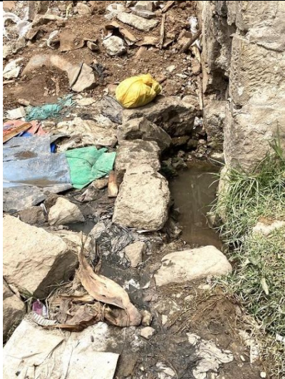
Water Leakage Point
