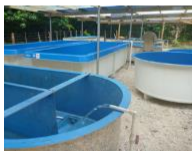
FRP tanks from Japan for newly installed
