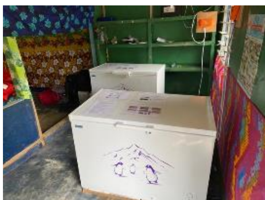
Solar freezer installation status
