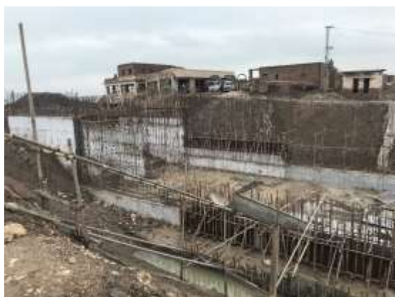
Photo 4.2.5 Situation of Danister Tail Regulator (1)
