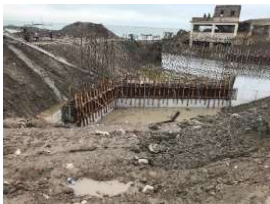
Photo 4.2.6 Situation of Danister Tail Regulator (2)
