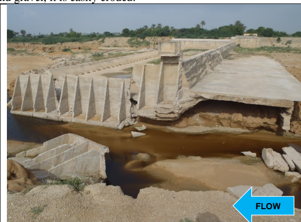
Malir Weir 1: Left side wall separated from main body
