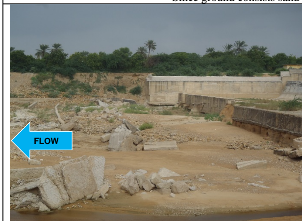
Malir Weir 1: Foundation of weir exposed due to lowered riverbed at downstream of weir
