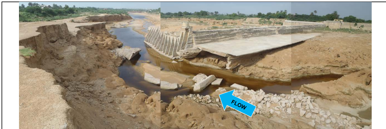
Malir Weir 1: Abutment section on the left bank has been destroyed. Since ground consists sand and gravel, it is easily eroded.
