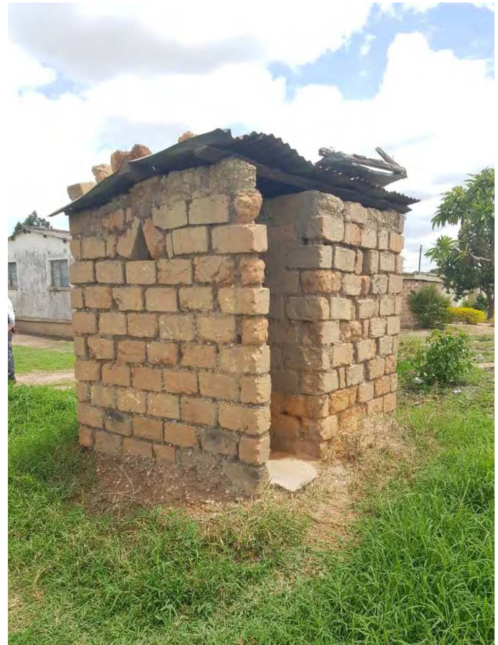
Poorly Constructed Pit Latrine
