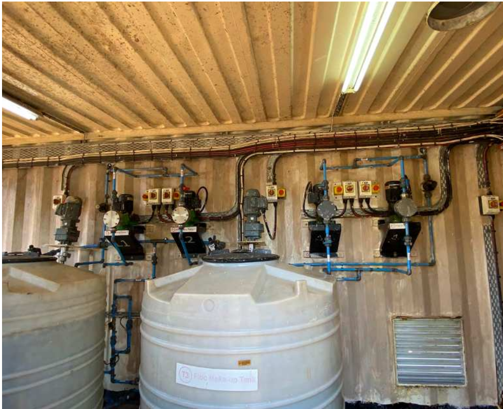
Water Treatment Facility
