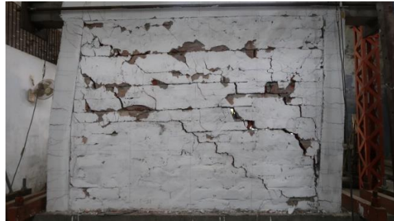
Pic.9 Failure pattern of a specimen tested by AUST, HBRI and TohokuU in Bangladesh (2018)
