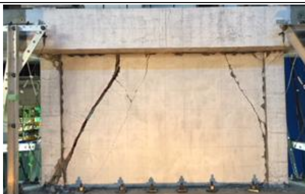
Pic. 21 Failure of a specimen with ferrocement retrofit
