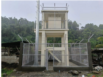
Outline of rainfall and water level gauging station
