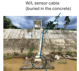
W/L sensor inside of maintenance box and protected with gabions
