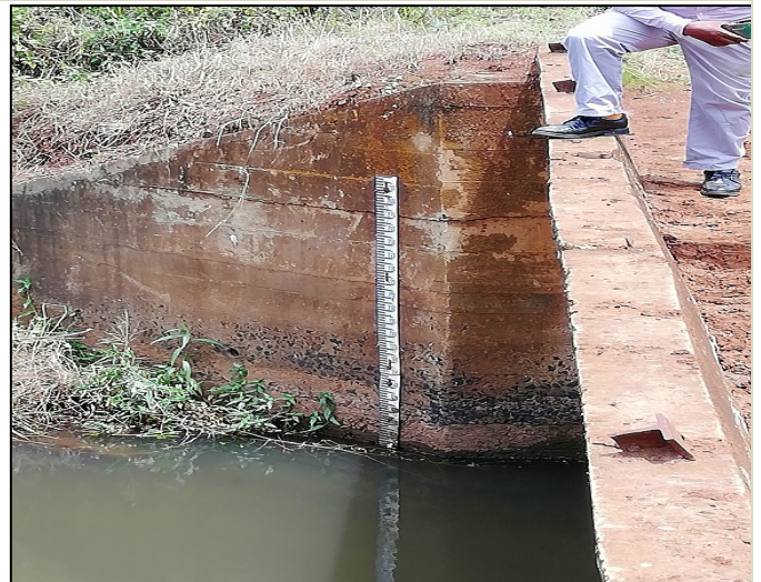
Site visit to Telemetering Station at 4DA11 Thiba. Staff Gauge for manual reading. (2021/10/26)
