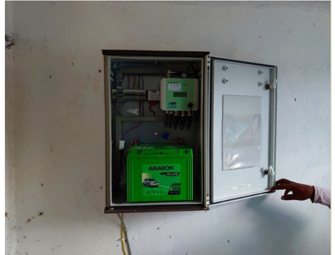
Site visit to Telemetering Station at 4DA11 Thiba. Telemetering Panel (up) and a car battery for power supply. (2021/10/26)
