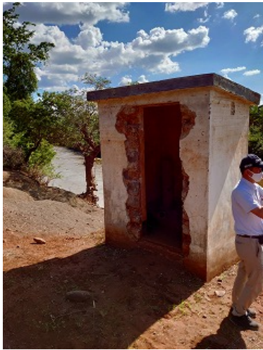
Telemetry Station in Tana Basin, 4BE10 Tana Rukanga. The door is broken with its concrete base and all the equipments are taken away. (2021/10/26)
