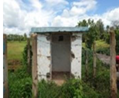
Photo 6: 4BB01 Station found vandalized. Staff gauge reading under the bridge was 1.10M at 1:06PM.
