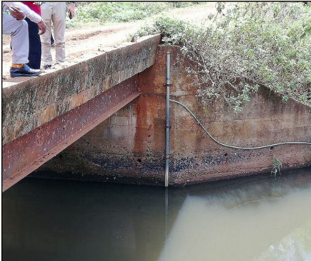
Site visit to Telemetering Station at 4DA11 Thiba. Outer view of the station building. Pressure sensor and cable. (2021/10/26)
