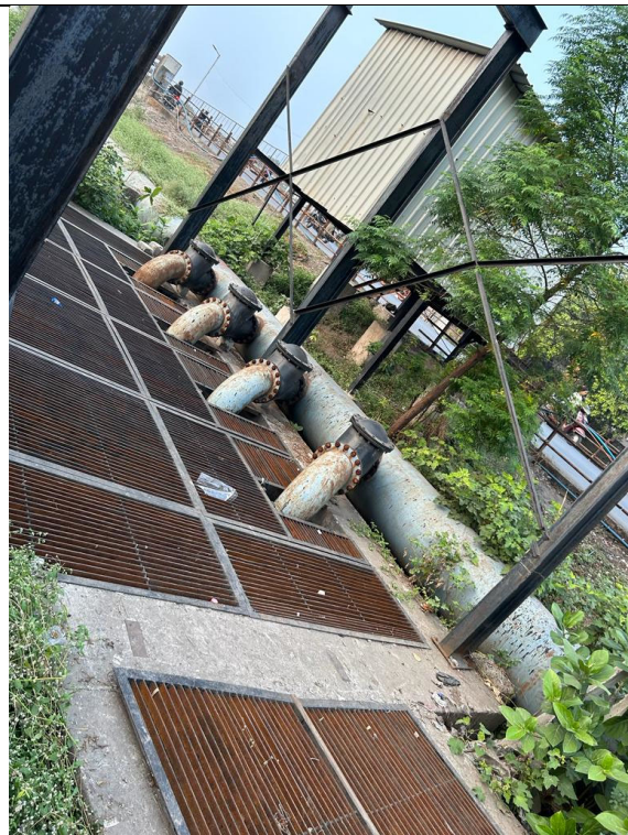
Pumps Installed in Meethi Creek Basin
