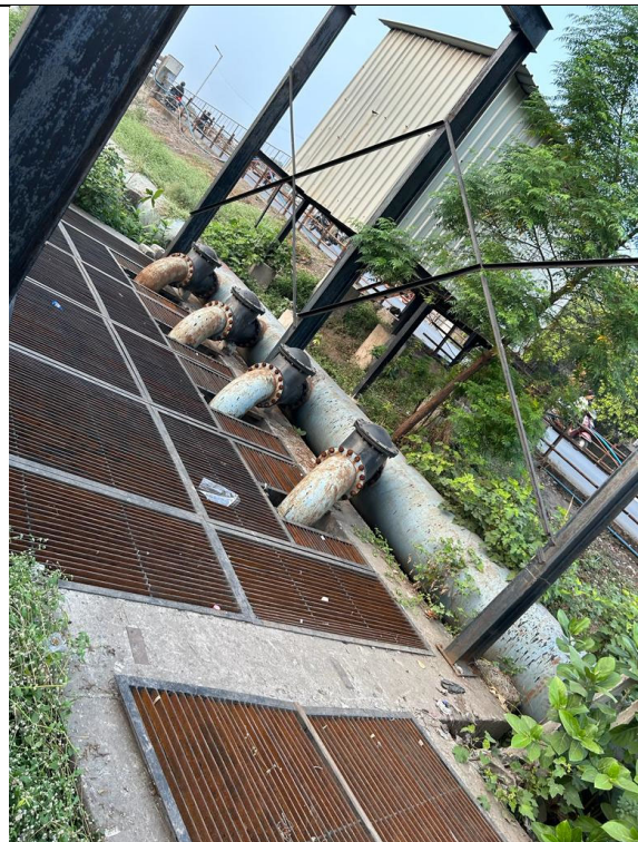
Pumps Installed in Meethi Creek Basin
