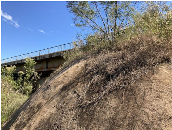
Trees growing on bridge revetment
