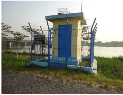
FFWS Installed Near Bojonegoro Barrage (Source: external evaluator)
