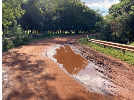
Gravel pavement section with water in the ruts
