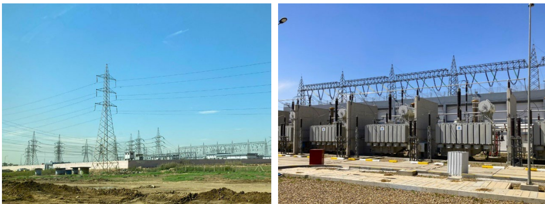
Newly constructed 400 kV substation (near Baghdad)
