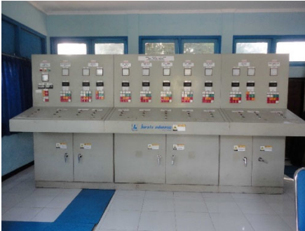
Water Gate Control Room of Bojonegoro Barrage (Source: external evaluator)
