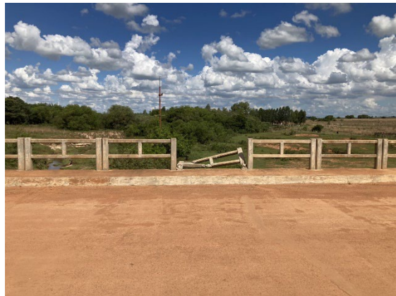
Damage to bridge fence
