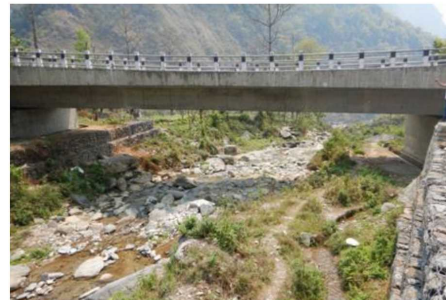
Photo 6: Gatte Khola Bridge (At the time of the post-evaluation, source: external evaluator)
