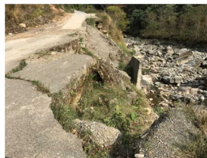
Photo 7: Location of collapsed approach road and a portion of the retaining wall at the Rangrung Khola Bridge. (Source: external evaluator)
