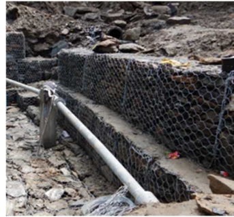
Photo 4: Holche system water pipeline (At the time of the post-evaluation, source: external evaluator)
