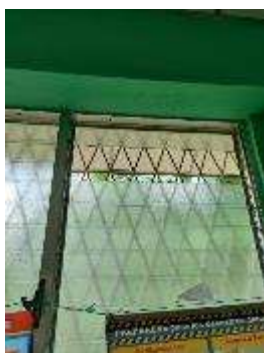
Photo 14. Missing Window Plates (Nueva Segovia)
