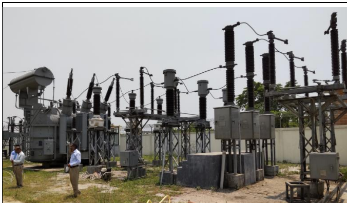
Training equipment (switchgears) within the substation premises
