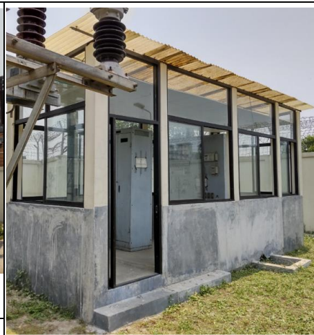
Training equipment (protection control device) within the substation premises
