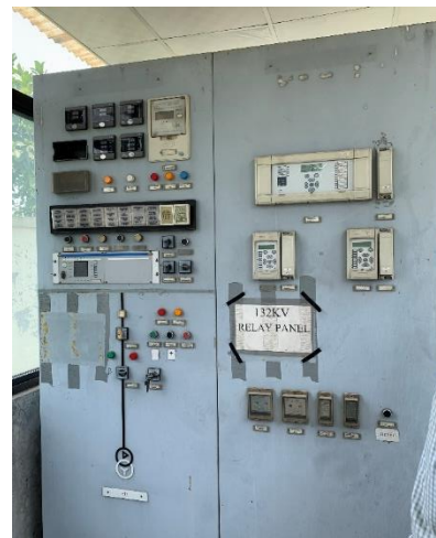
132kV relay panel
