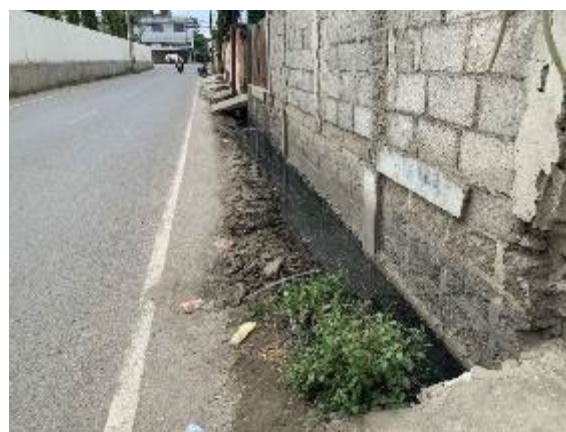
Status that Waste is clogged in the Gutter
