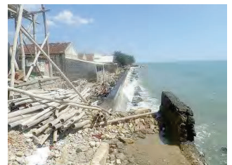
Coastal Condition at Down-drift Side
