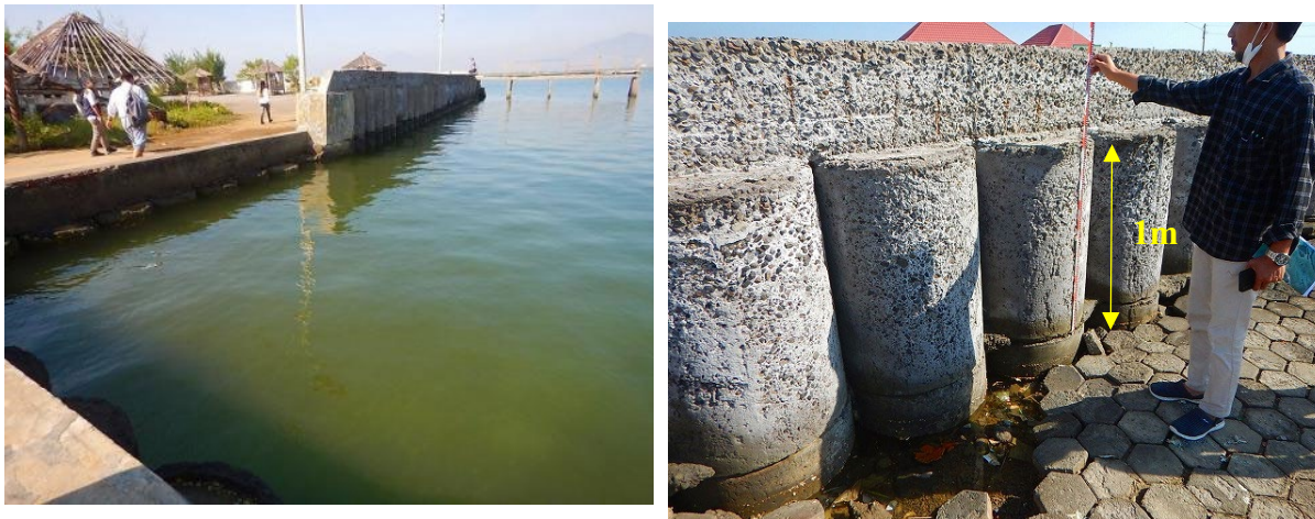
Photo 3 Seawall Condition (left) and Heightening of Seawalls (right)
