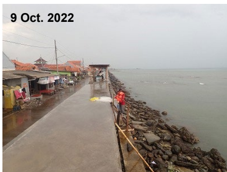
Coastal Protection at Urban Area (Line Protection) (Point P1 in the above figure)
