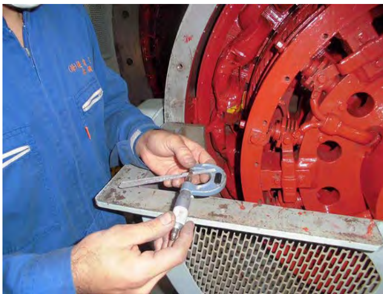
• Generator air gap Measurement
