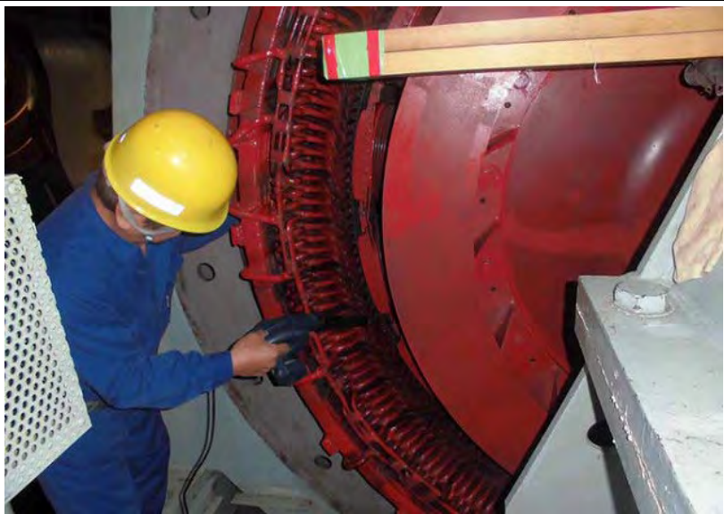
• Generator Air blow
