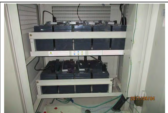
Pic 7-2 Backup storage battery
