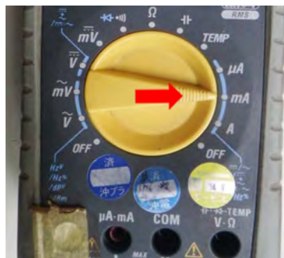
Current range (pressure transmitter, signal converter)
