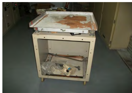
Circuit breaker rack
