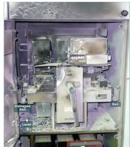
Damaged circuit breaker and position of level post-event
