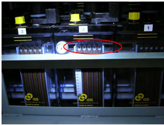
Photo1 Battery failure / Degraded matter
