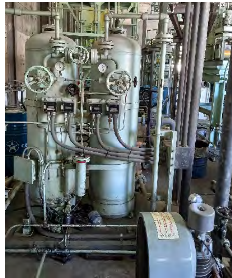
Picture 3. Air tank
