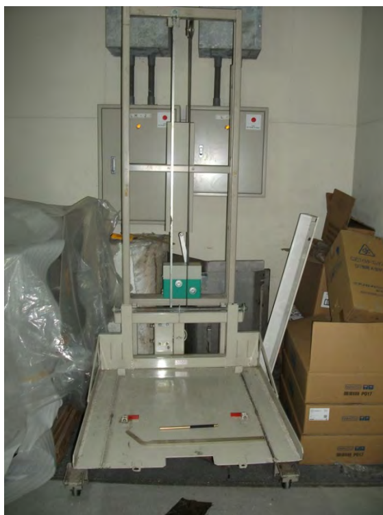
Circuit breaker lift
