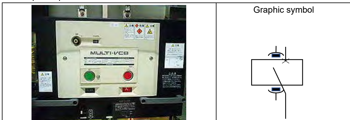
Pic. 4-2 Vacuum circuit breaker (VCB)
