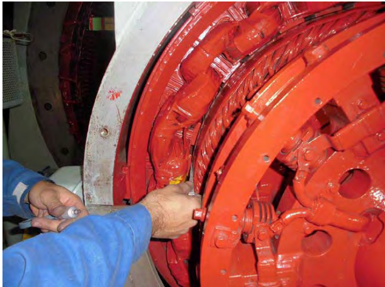
• Generator air gap Measurement
