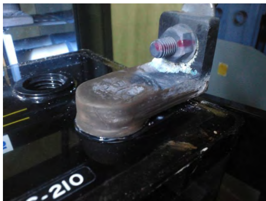
Photo3 Battery failure Terminal attachment
