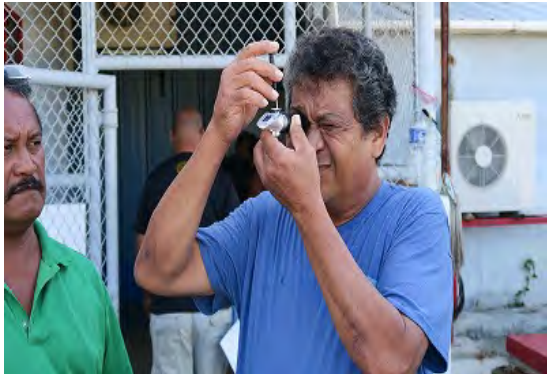
05-Inspection of batteries(specific gravity)
