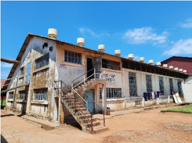
The building of a ginnery whose base was constructed in the 1920s
