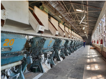
Old ginning facility which requires constant maintenance
