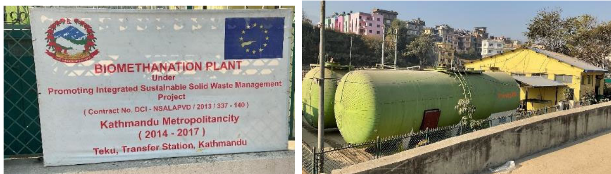
Figure 3-16 Methane Gasification Facility in KMC
