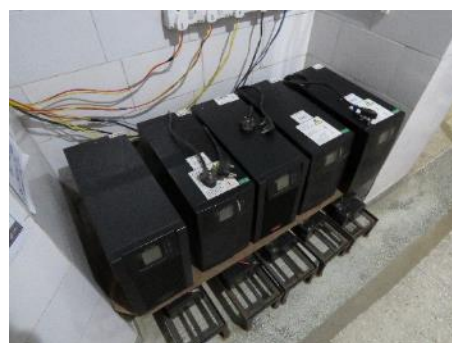
Batteries (One for Each Dialysis Machine) in Case of Power Failure
