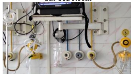
Central Medical Gas Supply Outlets
