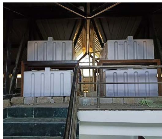
Overhead Tank of 100-sqm Apartment
