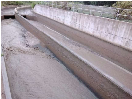
After Sand trap maintained clean Feb 2023, Same location from upper stream
