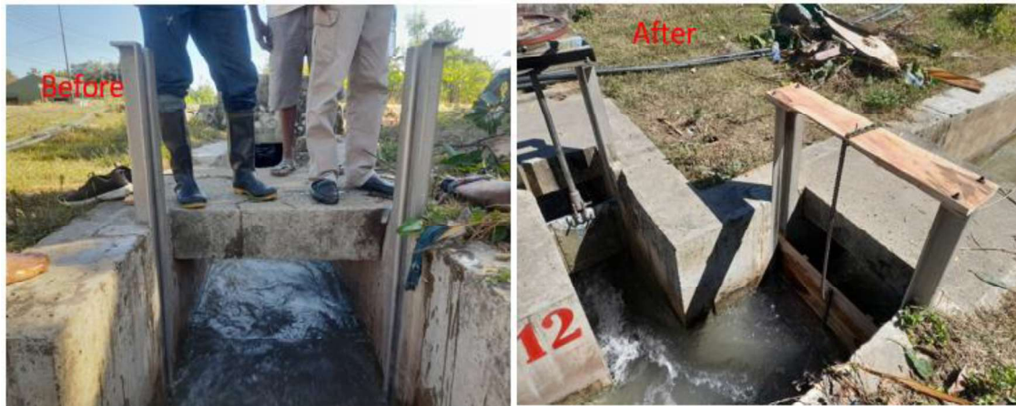
New stop log installed at OT 12 in Maliana1 IS
