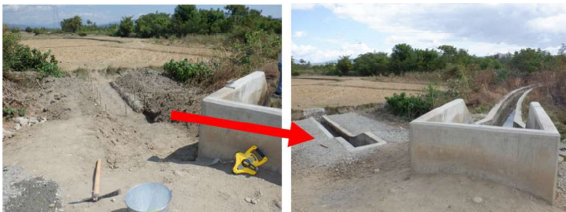
New diversion facility for Bibiten (OT 5) and Garemarak (OT 6) in Buluto (left-hand side: before, right-hand side: after)
