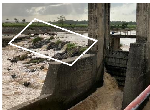
Aglipo 2 water intake point. There used to be a rubber dam on the right bank side of the flood discharge gate (white frame), but it is no longer
