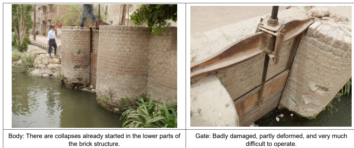
Figure 4.4.9 An Example of a Status S1 Structure, Reassessed from the 1 st Stage Survey Result
