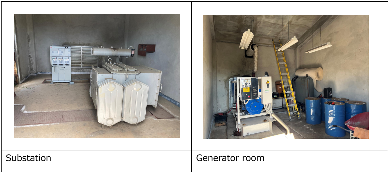
Figure3-2-8 : The picture related to Emergency Diesel Engine Generator
