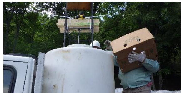
Photo 16. Agitator installed on top of tank
