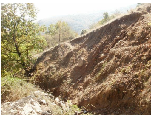
Photo 9: Place with advanced erosion, where installation of a gully plug is considered
