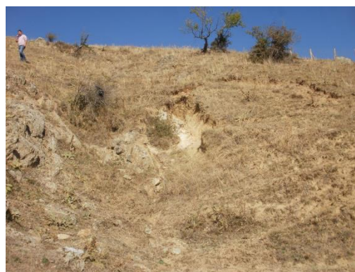
Photo 10: Place with advanced erosion, where installation of a gully plug is considered
