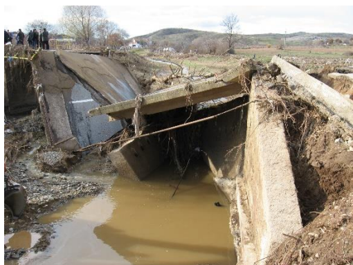
Photo 1: A bridge destroyed in 2008
