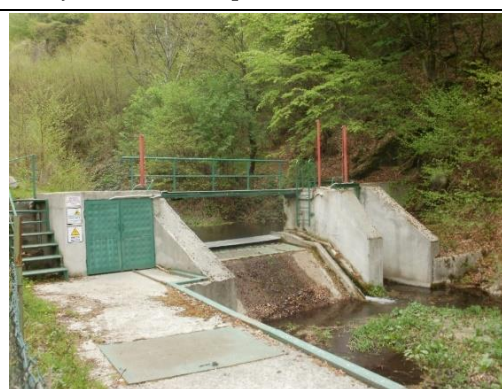
Photo 5: Ljubanci small hydropower facility (Forest compartment No 90)
