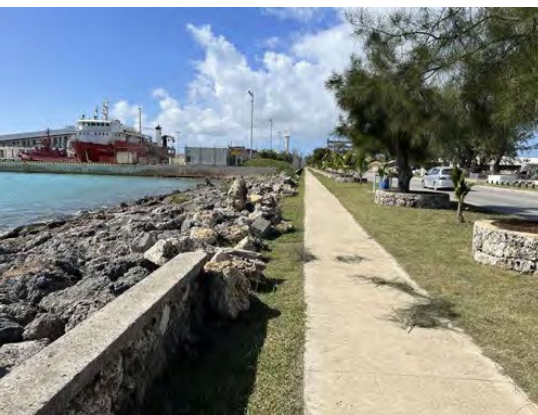
Photo 4.1.15 Collapsed part about 45m from here
