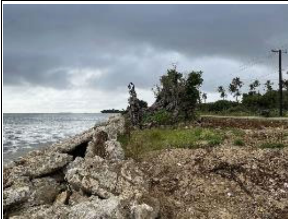
Photo 2.7.13 Destroyed Concrete Coating
