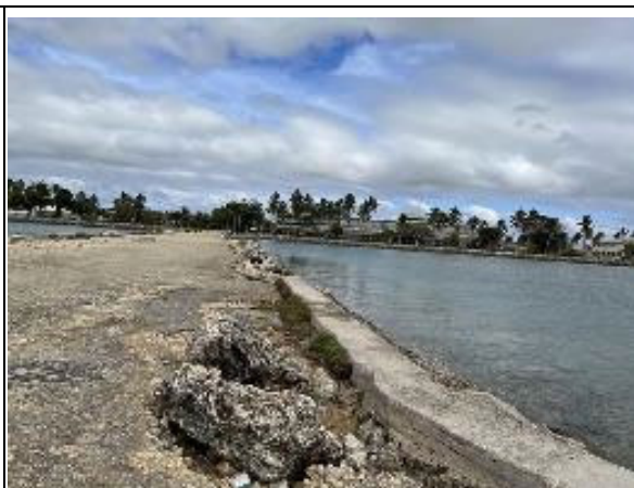
Photo 2.7.8 Damage on the West Side of the Jetty
