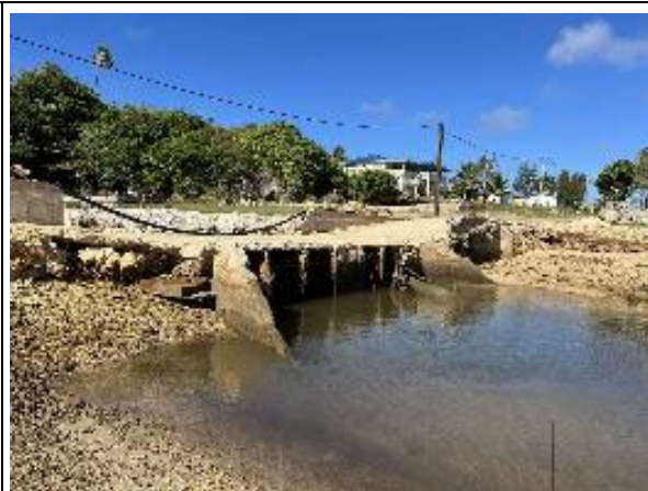
Photo 2.7.22 Damaged Bridge (Culvert)
