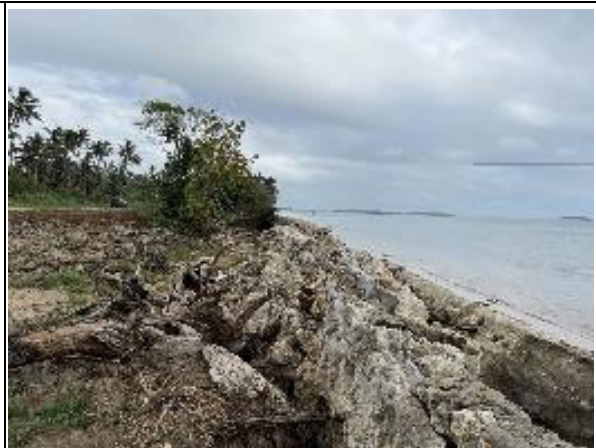
Photo 2.7.12 Destroyed Masonry Seawall
