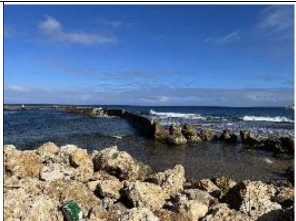
Photo 2.7.18 Masonry Breakwater has Collapsed
