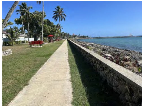
Photo 4.1.12 The seawall is partially maintained.
