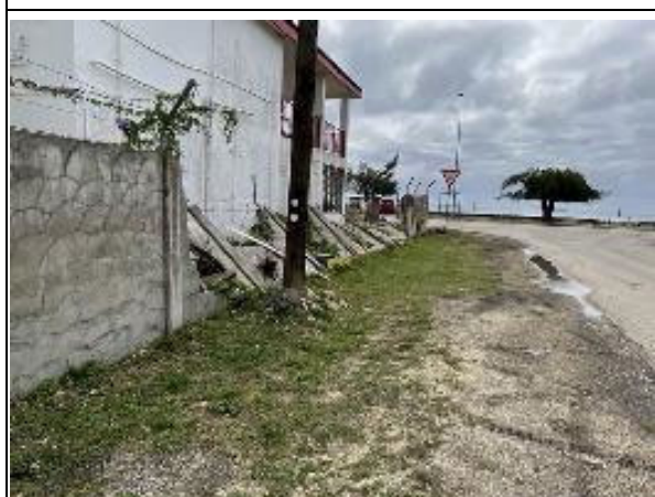
Photo 2.7.9 Block Wall Destroyed by Tsunami
