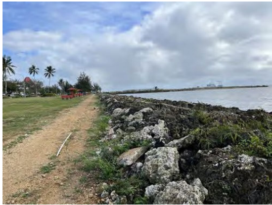
Photo 4.1.11 Seawall collapsed at Vuna Wharf
