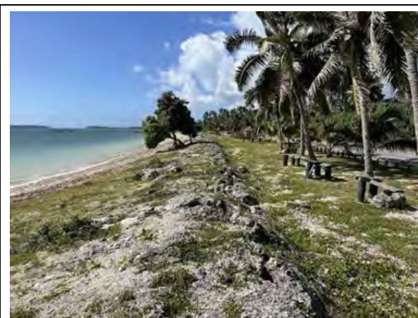
Photo 4.1.8 This can no longer be called a seawall.
