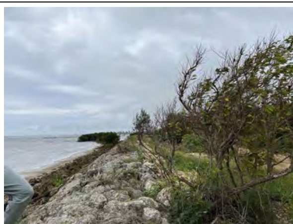
Photo 4.1.2 Damaged masonry seawall by tsunami
