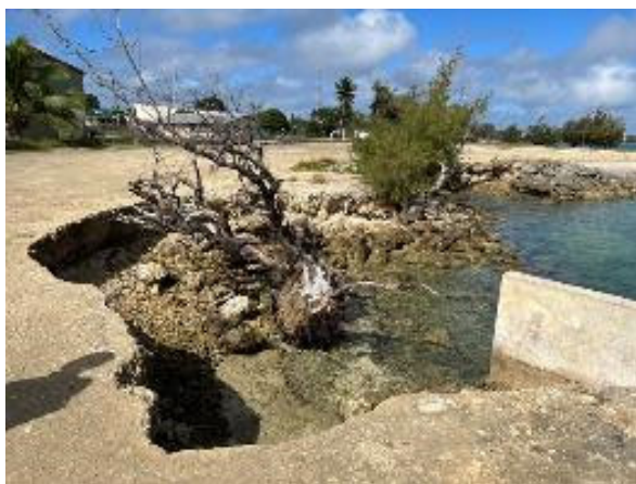
Photo 2.7.33 ⑨Scouring bottom of the slipway
