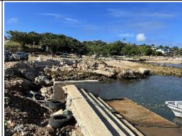
Photo 2.7.20 Damage to Small Vessel Wharf
