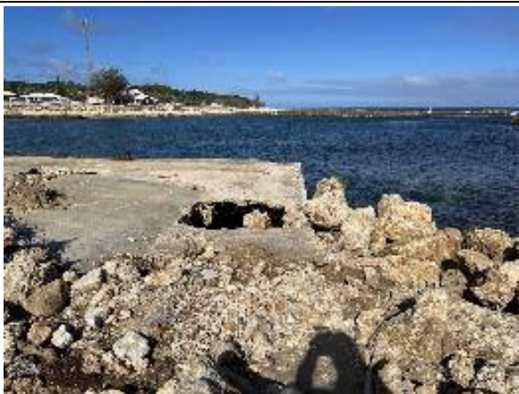
Photo 2.7.19 Damage to New Port Apron
