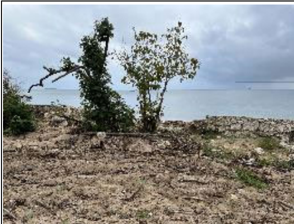
Photo 2.7.11 Condition of Masonry Seawall after the Tsunami
