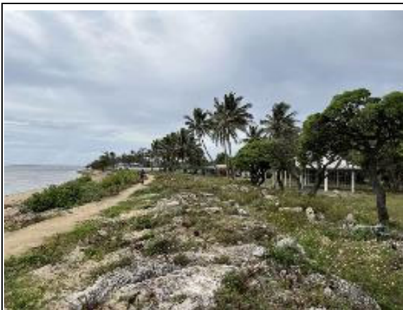
Photo 2.7.5 Scattered Stones on Masonry Seawall
