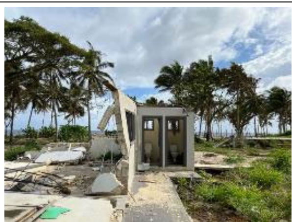
Photo 2.7.2 Building Destroyed by Tsunami
