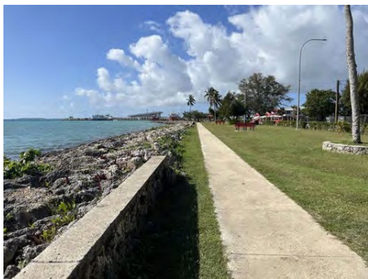
Photo 4.1.13 Damaged part from here
