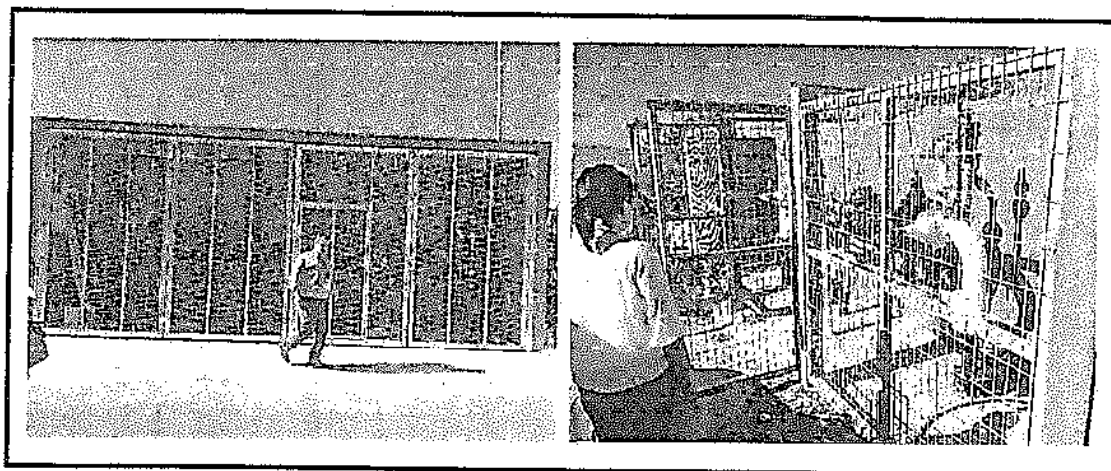
Pressure Reducing Valve (photos in JSC, Jenin)
